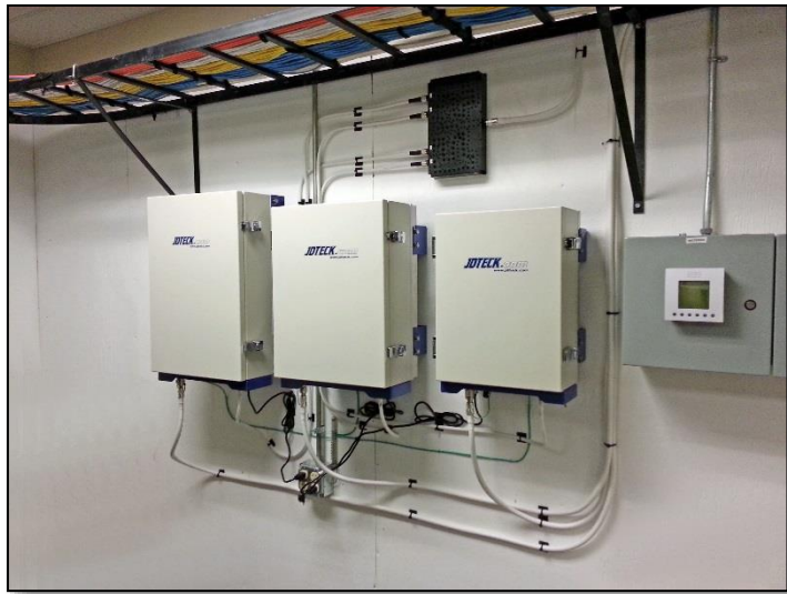
Example of repeaters installed in communications closet.
